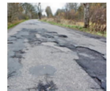
Parking near uneven roads
